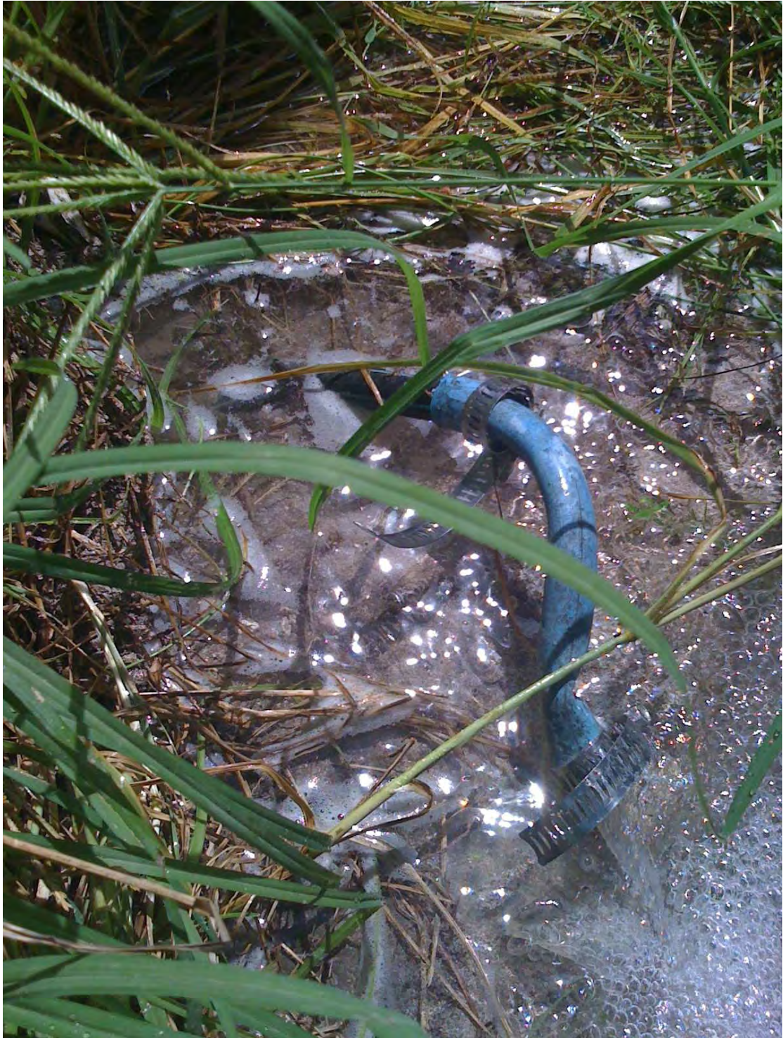
A severed 90 degree connection on disused but still connected line. Years of ground pressure forced the connection to snap at the elbow.
