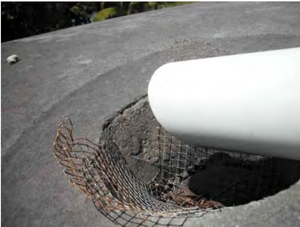
A1.2.2 Makeshift entry screen on ferro-cement tank.
