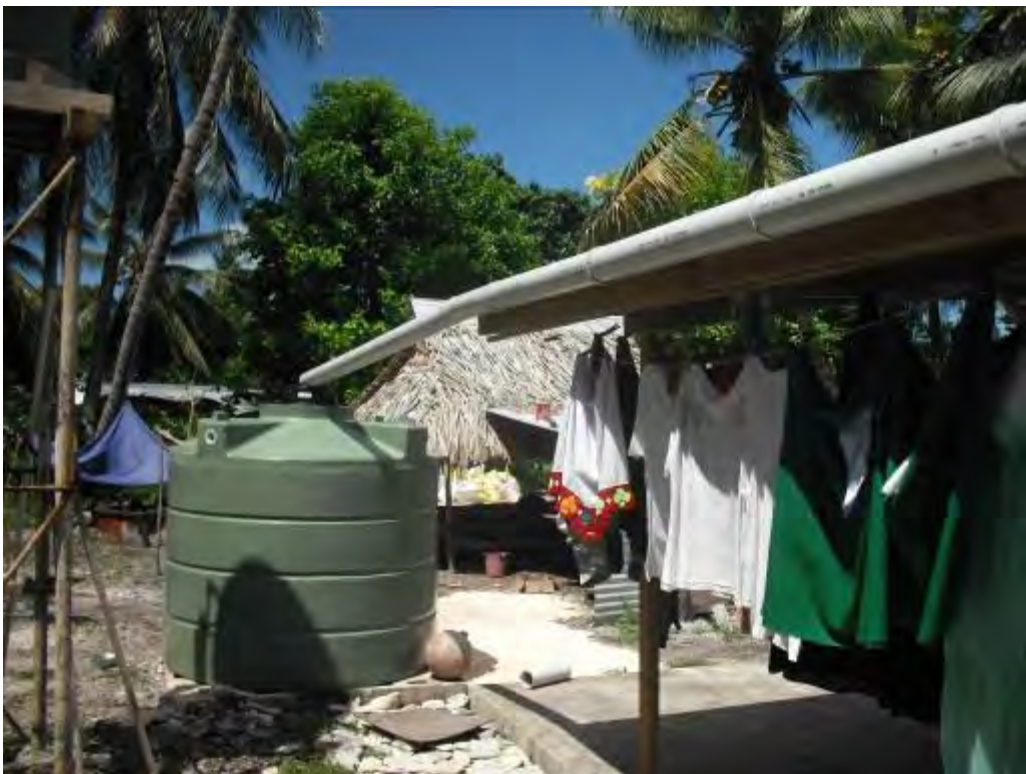
A1.1.9 Split PVC guttering, well supported. Unsupported downpipe to new polytank.
