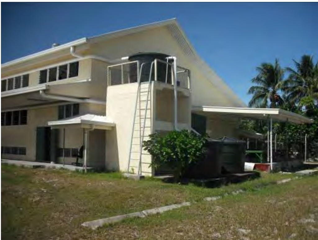
A1.4.2 Well designed and constructed collection, transmission and storage system. Overflows routed to a soakaway. Unfortunately, collected water is not fully utilised. There is no ownership of the water at Government buildings.
