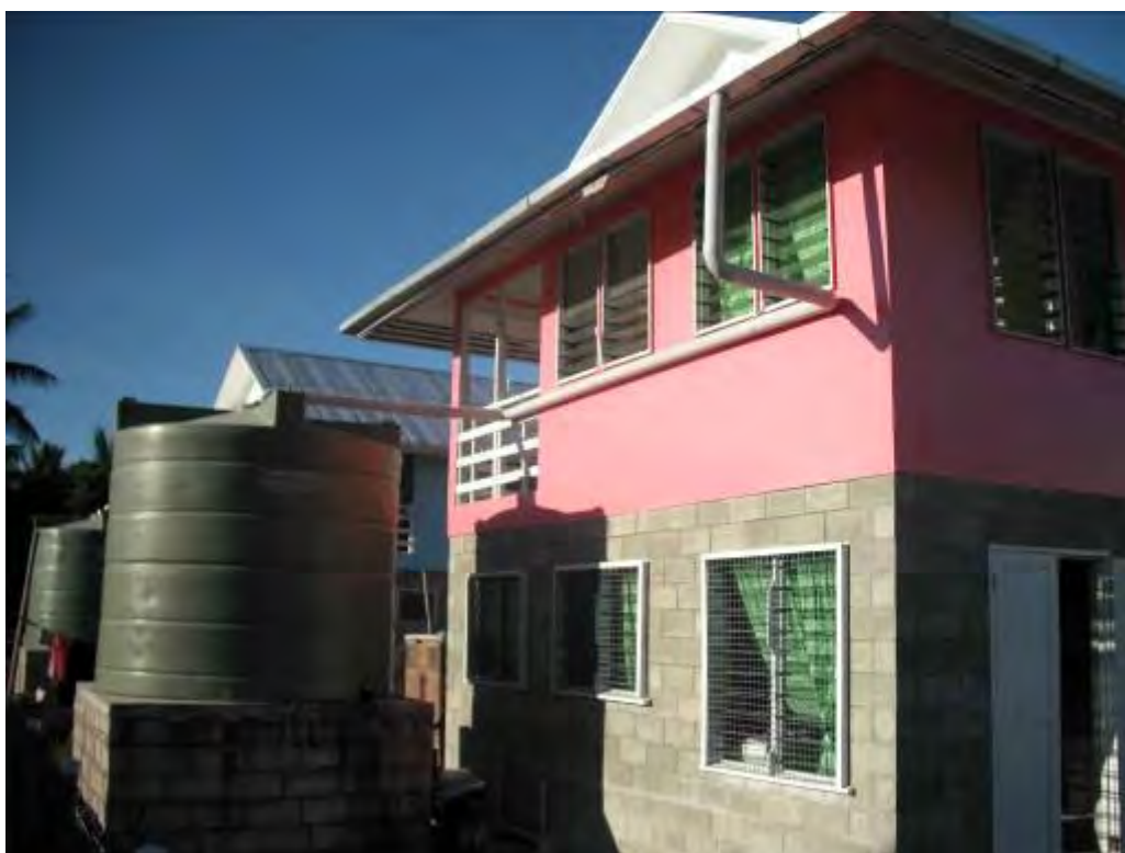
A1.3.8 Elevated 10KL polytank to utilise potential energy provided by high roof eaves.
