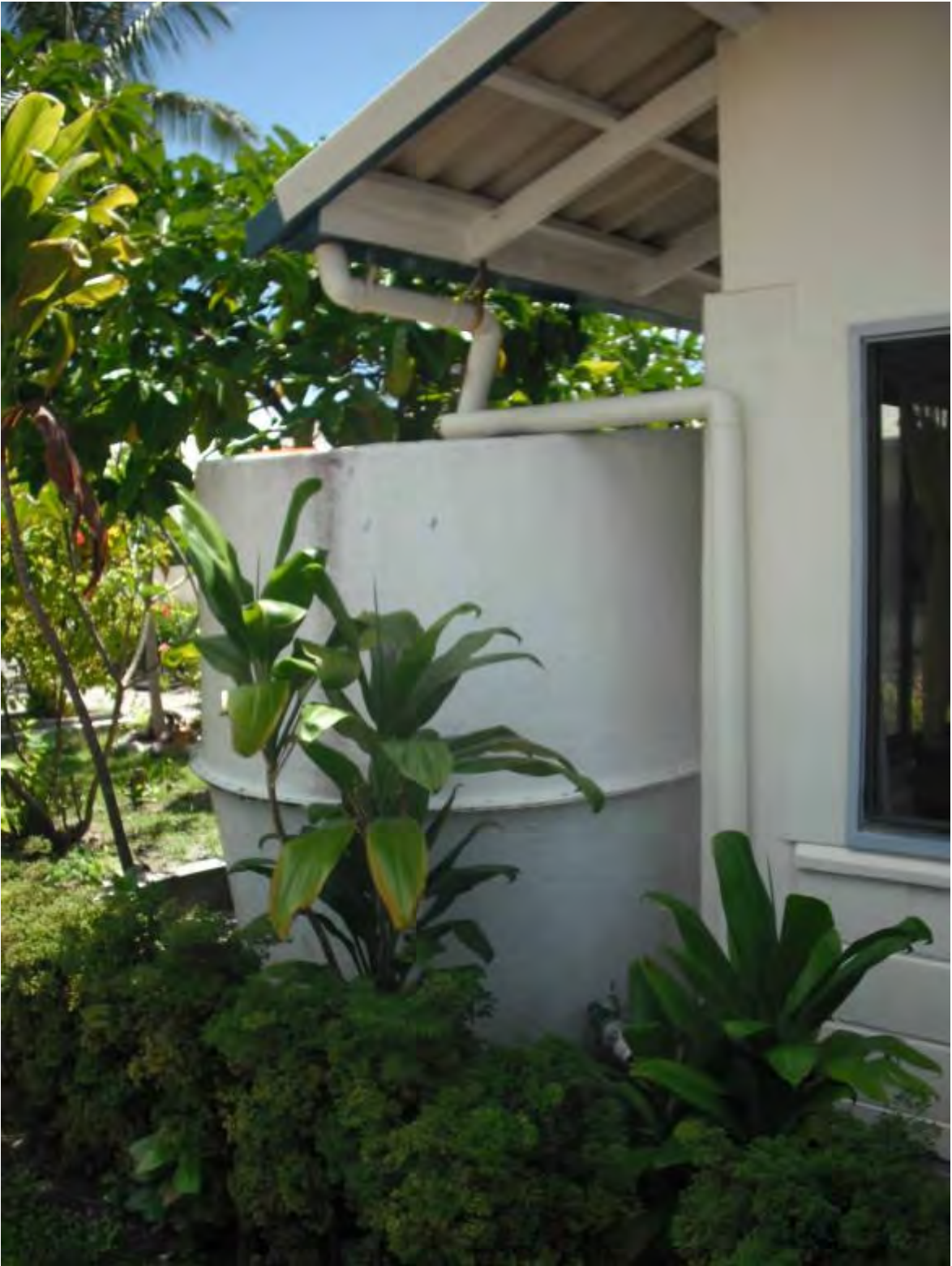
A1.3.5 Two piece fibreglass tank.
