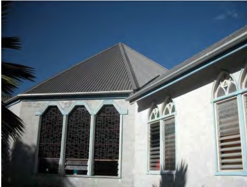
A1.1.14 Large roof catchment area with inadequate gutter or downpipe size. Limited fall on gutter.
