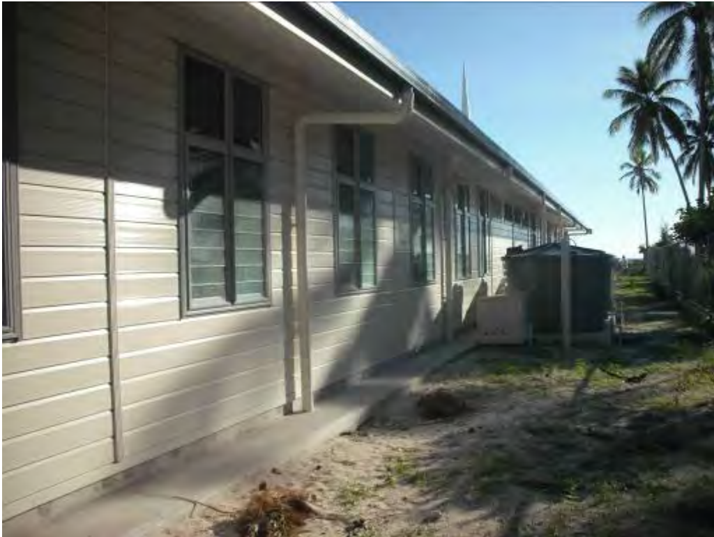
A1.4.1 Well constructed guttering system with adequate downpipes, underground transmission and significant storage in connected polytanks.
