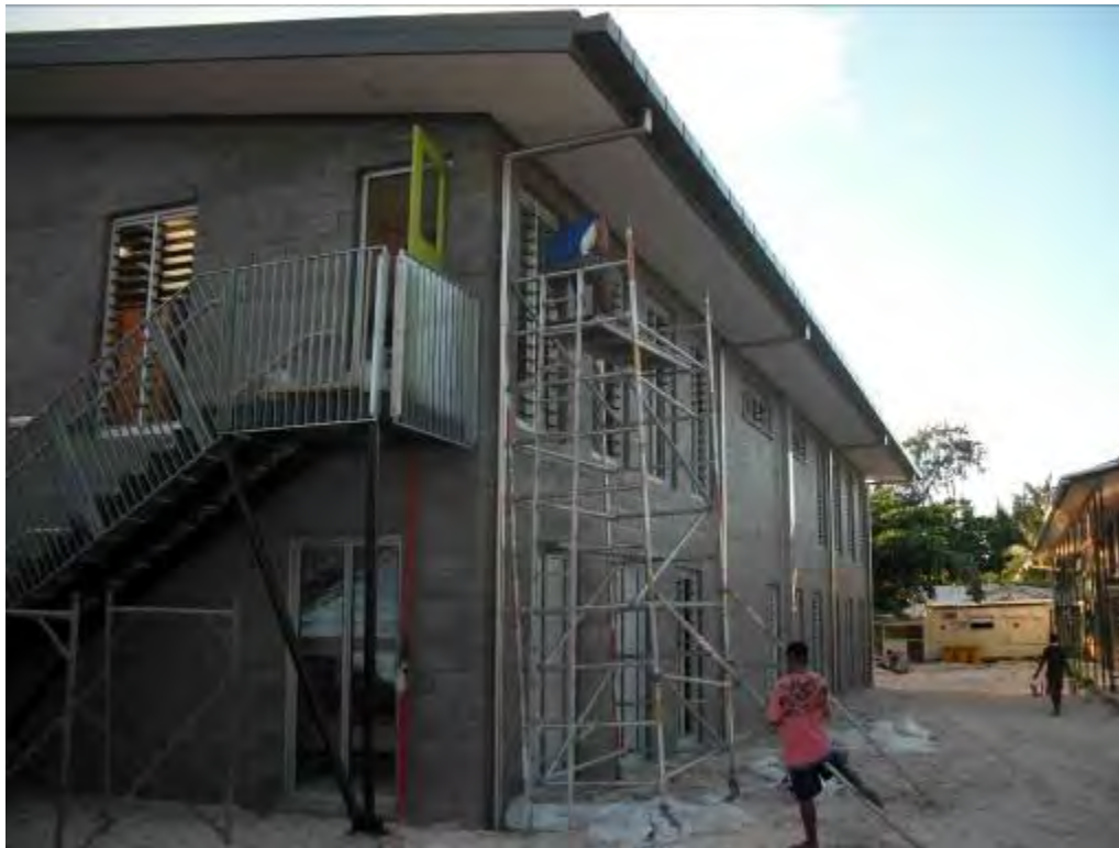
A1.1.3 New zinalume ® guttering and stainless steel downpipe to underground PVC transmission pipes to multiple 25KL polytanks being constructed. Downpipes are well supported.
