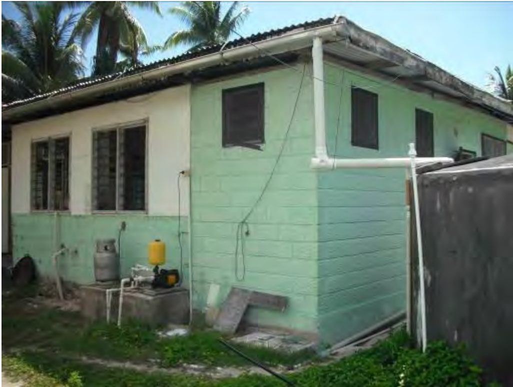
A1.1.8 Small cross-section PVC gutter suitable for small roof area, single unsupported downpipe (liable to failing) to ferro-cement tank.
