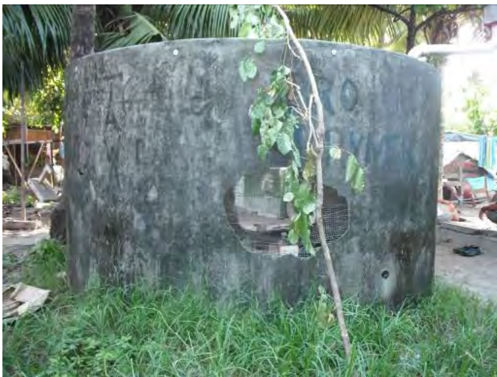
A1.3.7 Neglected 10KL ferro-cement tank
