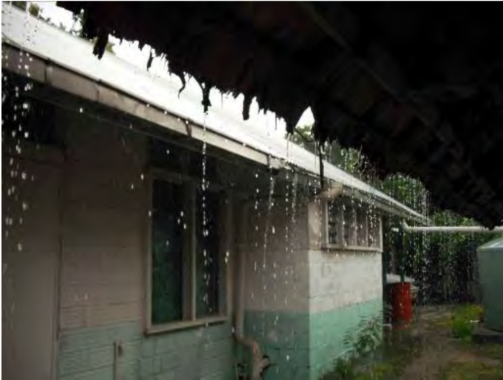
A1.1.21 Incomplete, poorly maintained gutter system unconnected to downpipe. Unsupported downpipe. Thatch roof in foreground unsuitable for rainwater collection.
