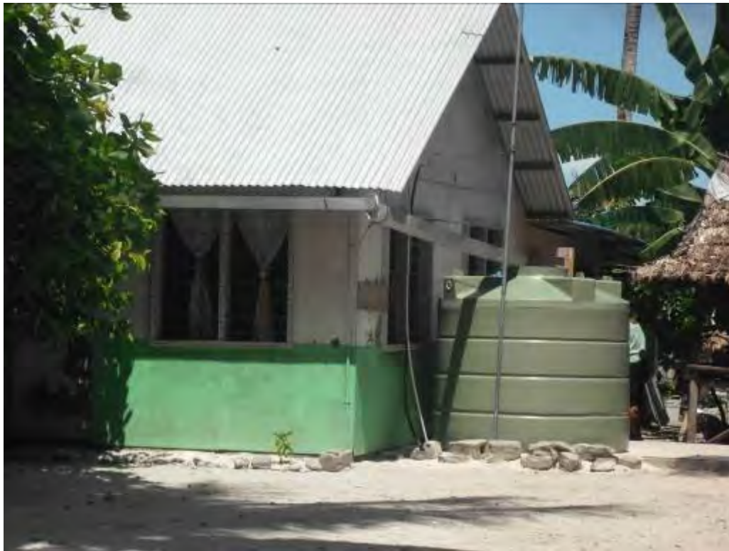
A1.1.10 Poor makeshift guttering and makeshift transmission to brand new polytank.
