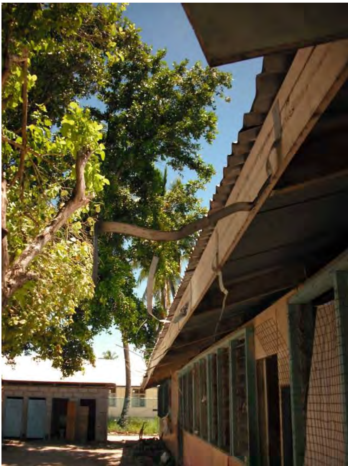
A1.1.5 Guttering missing, poor maintenance. Overhanging trees.
