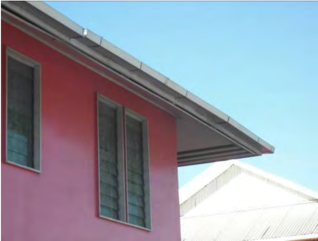
A1.1.16 Newly fitted gutter already broken, and inadequate fall. Poor materials and installation technique.
