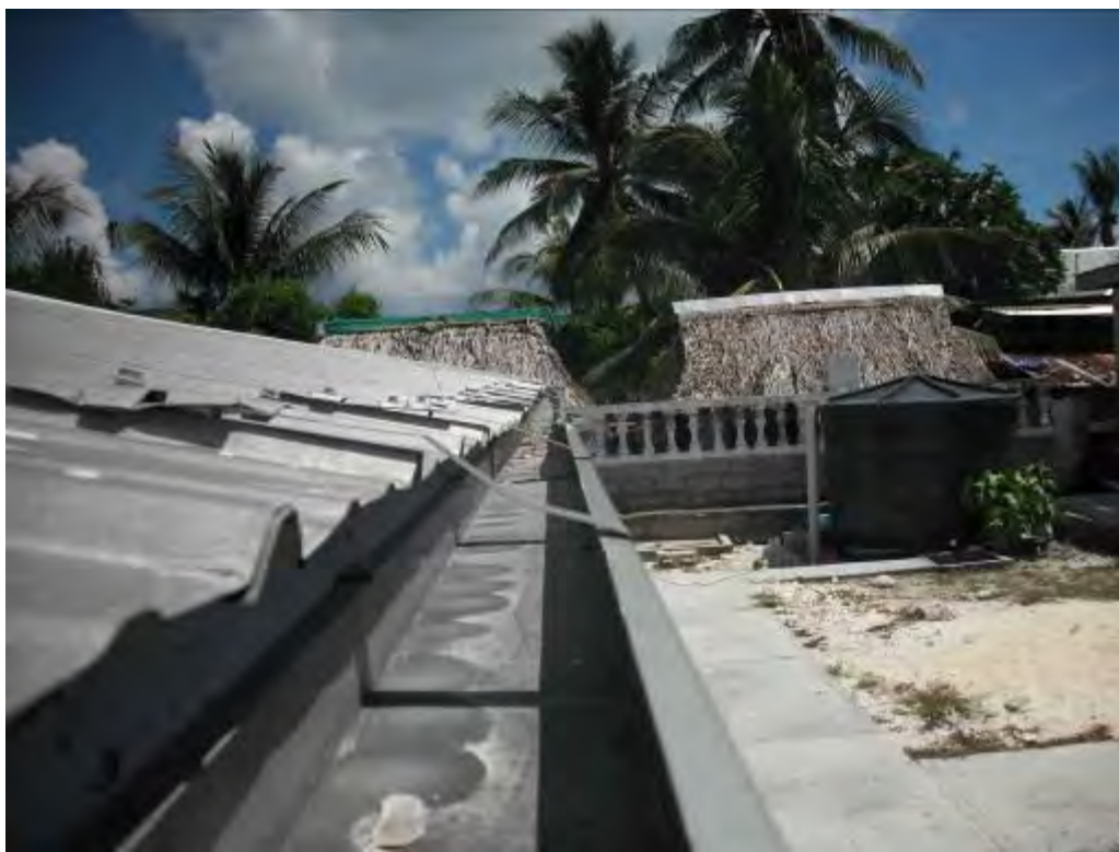
A1.1.1 Well supported galvanized steel maneaba guttering, fairly clear of debris, Infrequent downpipes to underground transmission.
