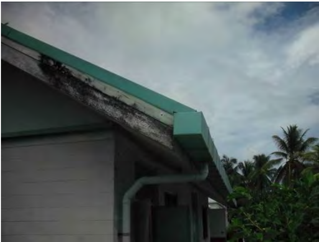
A1.1.20 Large cross-section gutters and well supported downpipe to underground transmission. System in place for c. 20 years but well maintained.
