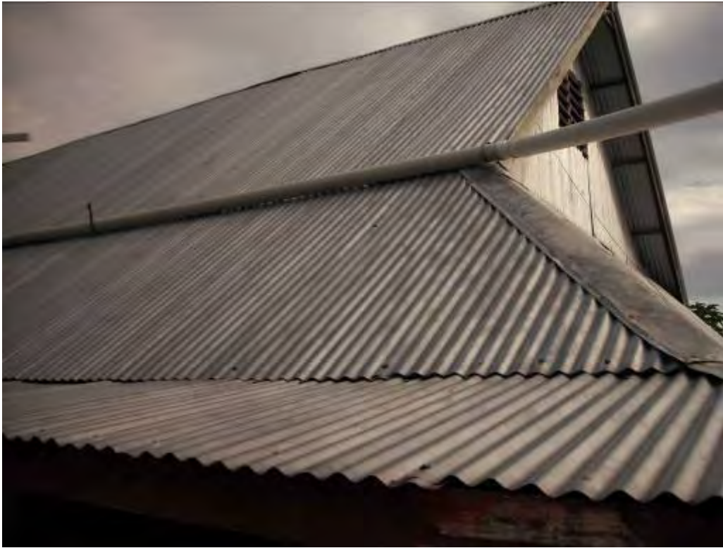
A1.1.19 Split PVC gutter half way up maneaba roof. Unsupported downpipe liable to fail.
