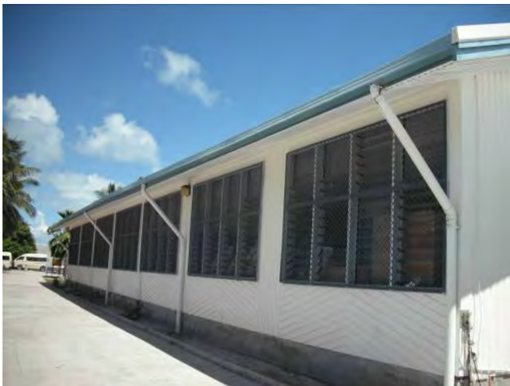
A1.1.11 Good sized gutter (with high outer wall to reduce splash losses) with adequate downpipes to underground transmission. This system is old ( c. 15 years) but well maintained.
