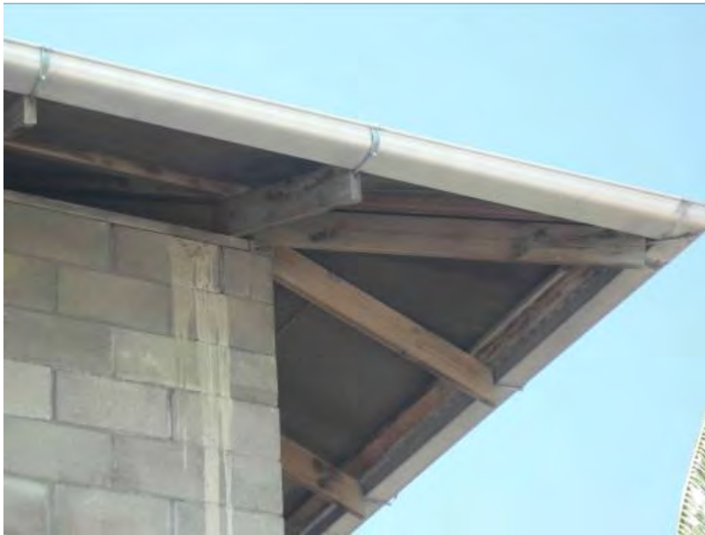
A1.1.6 Small cross-section PVC guttering at a primary school, not suitable for this large roof catchment with inadequate downpipes
