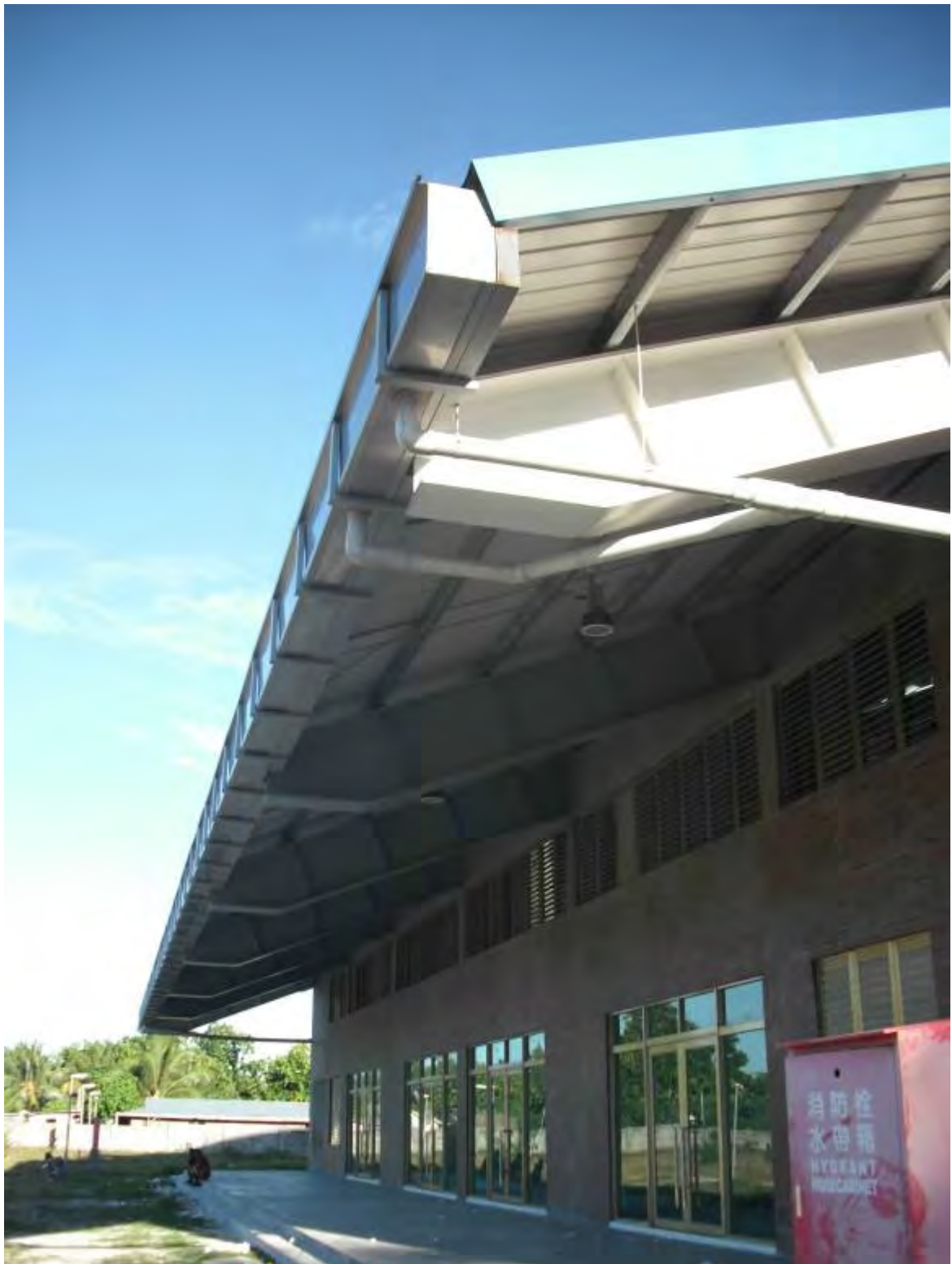
A1.1.18 Newly fitted very large cross-section gutters and large diameter downpipes to accept water from a large roof catchment. Water routed underground to large reinforced concrete cistern.
