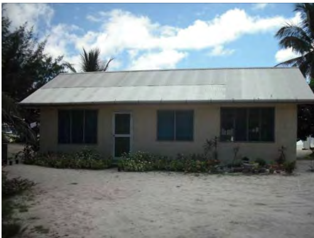
A1.1.2 Split PVC pipe guttering. Well supported and with a fall towards the downpipe. Good clean roof catchment for collection with no overhanging vegetation.
