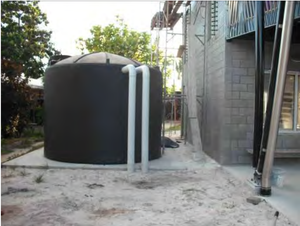
A1.3.1 Large imported 25KL polytank on flat reinforced concrete slab
