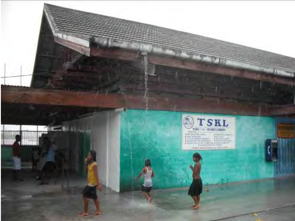
A1.1.22 Large cross-section gutters, missing downpipe.
