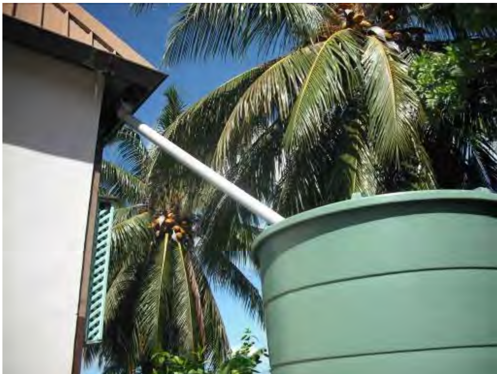
A1.1.4 V-shaped galvanised steel guttering. Government owned hotel. Inadequate for large roof area, makeshift unsupported downpipe to polytank.
