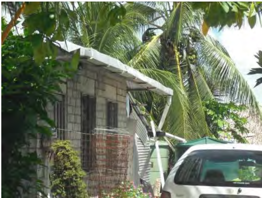
A1.1.7 Large cross-section makeshift guttering. Made from folded galvanised iron sheet. Unsupported downpipe, liable to fail.
