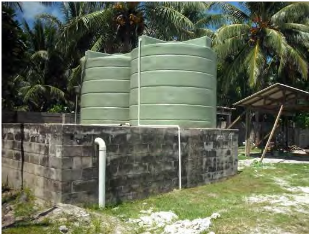
A1.3.4 Large semi-submerged block work cistern, with pumped elevated storage in 2 No. 10KL Poly tanks.
