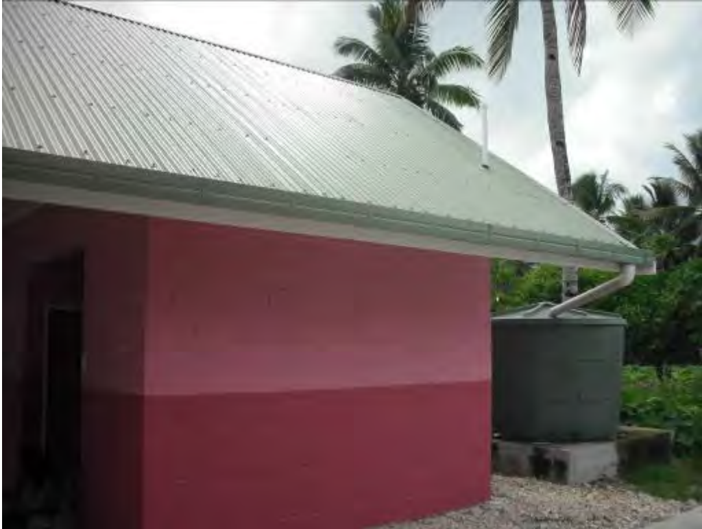
A1.1.17 Newly installed gutter, downpipe and tank. Well fitted but downpipe not secured so liable to failure
